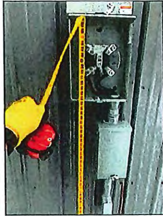
Meter installed 3 feet 6 inches to 5 feet above final grade.
