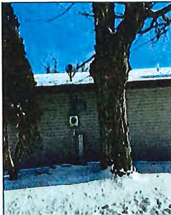
Approved overhead service, meter set only.
