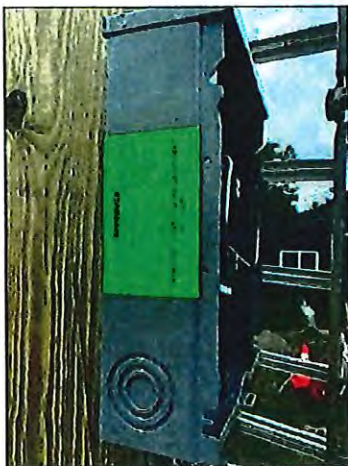
Meter socket inspection sticker.
