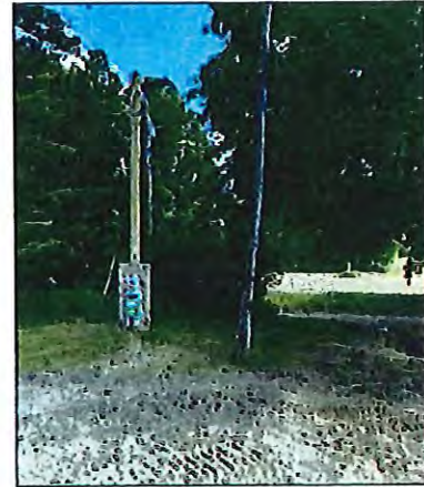
Approved overhead temporary service and a clear path.
