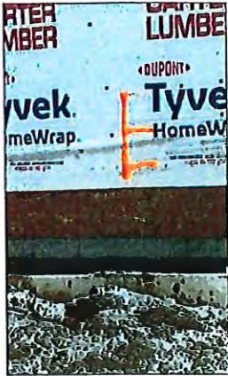
Meter location marked.
